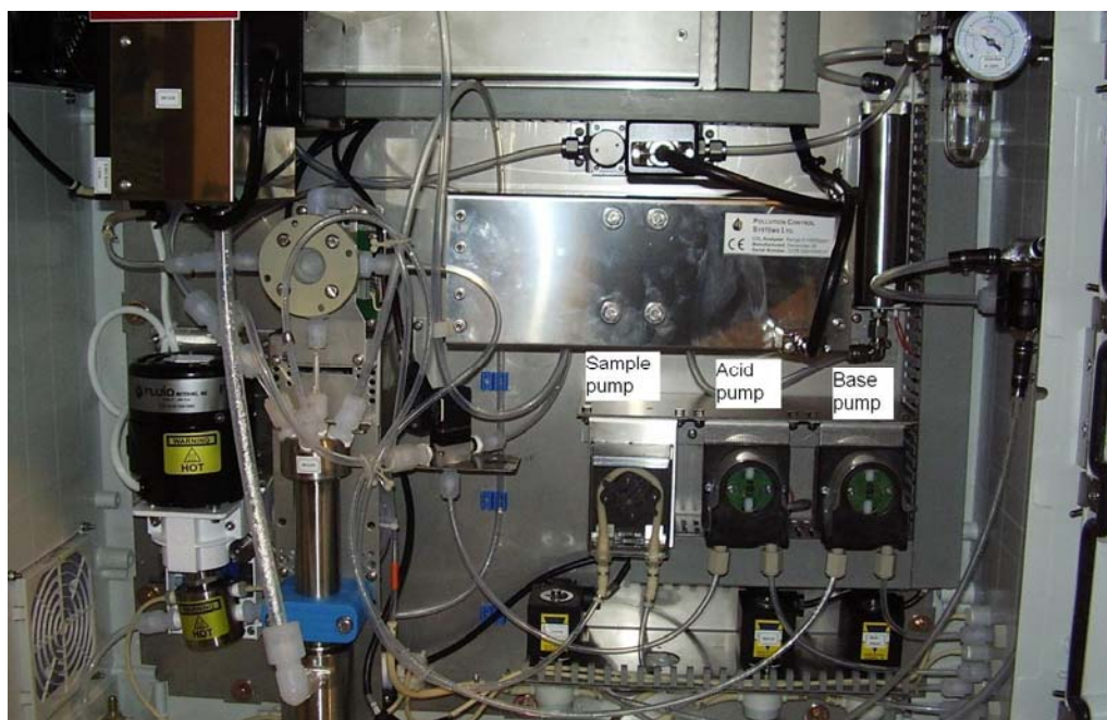
Location of Sample, Acid and Base pumps.
